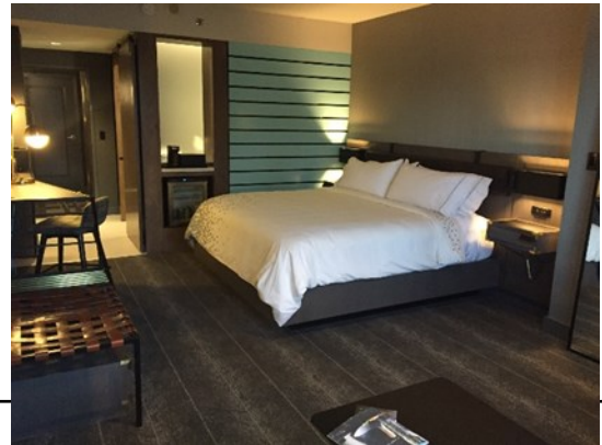
The Siena Hotel is well on the way to becoming the Renaissance Reno! The model room (above) gave the team a glimpse into the future of the hotel, and the exterior paint scheme (below) is beginning to take shape. The interior Bocce Courts are under construction, turning the 10,000 sq ft space into an entertainment haven! Conversion to the Renaissance Reno is schedule for January 2017.
